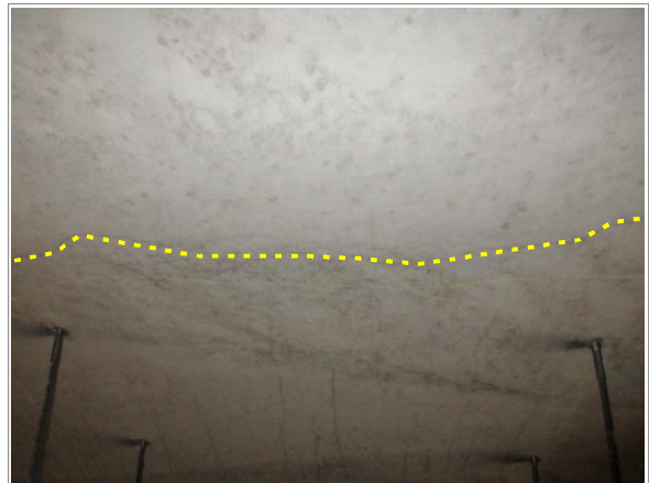
Span61 천단부 균열(cw=0.3mm/9.0m)
